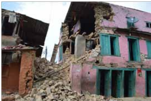
Partially collapsed stone rubble masonry buildings along Tribhuvan highway (photo: Sujan Malla)
