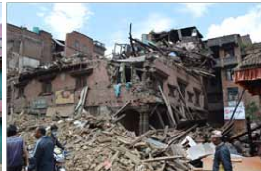
Brick masonry buildings with collapsed upper storeys in Bhaktapur (photo: Sujan Malla)
